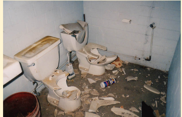
Vandalised toilet compartment
